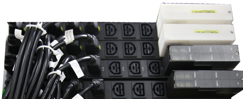
Figure 6-6 Horizontal PDU power cable and PDU
